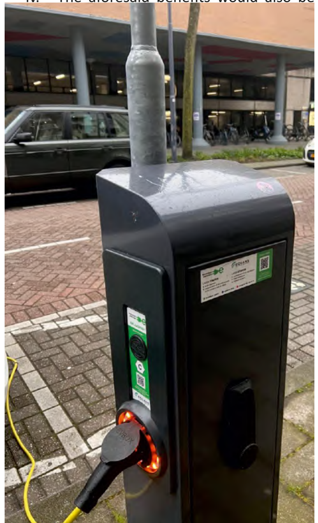
EV Charging Station
