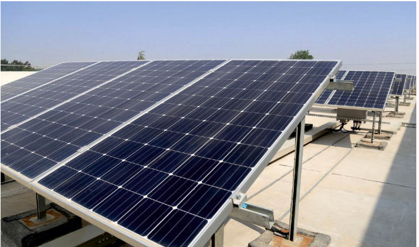
Solar Rooftop Plant
