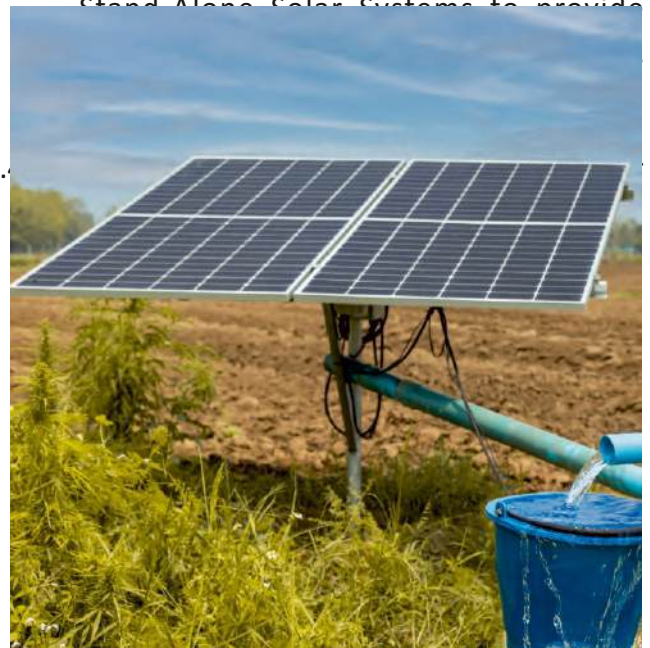
Off Grid Stand Alone Solar Pump
